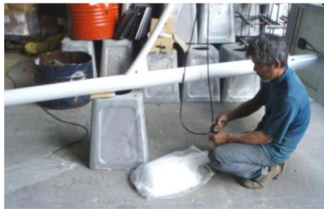
Lamp (Light-1、Light-2) Cable connect to (Light-1、Light-2) Cable
